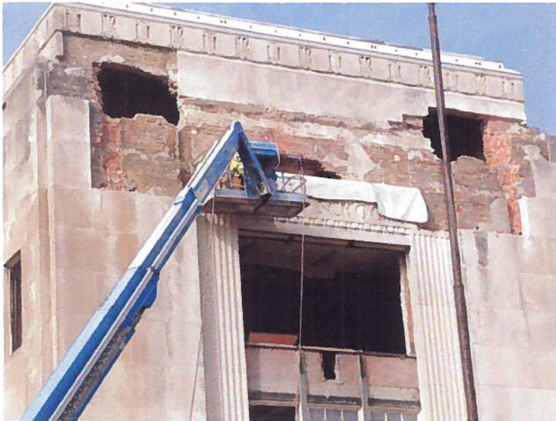
Demolition crews razing the old John Marshall High School first extracted ornamental features of the building, such as stone medallions, so they could be preserved for future use. The holes in the structure show where the stone relief was removed.
